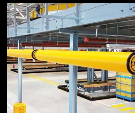
Multiple Alarm Bar safeguarding an overhead structure.
