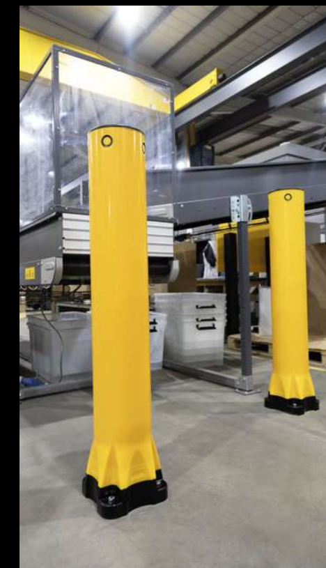
190 Monoplex Bollards defending critical equipment in a manufacturing facility.
